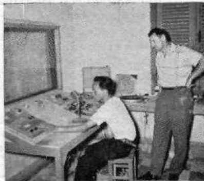
The New Recording Studio during Installation
